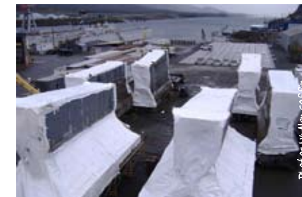
Blocks and modules waiting to be moved to the pad for ship erection.
