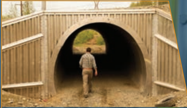
Hawk Lane: $2 million, upgrade Hawk Lane from Victor Road to school entrances. Commuter culvert installed.
