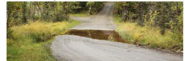
Figure 1 - The low area where water is across the roadway is the location of the rock fill drain.
