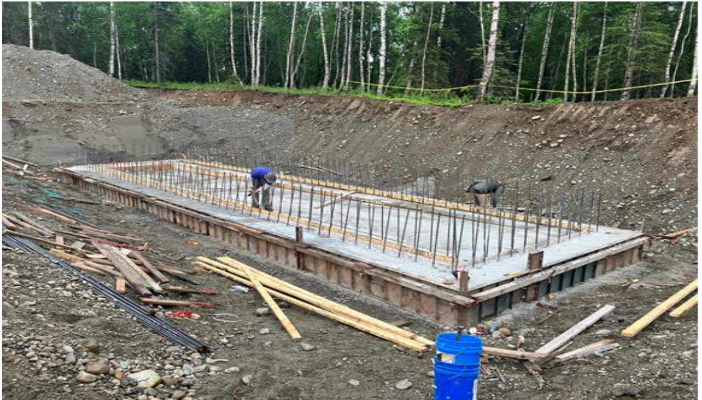
Above photo: Fire Water Storage Tank Base
