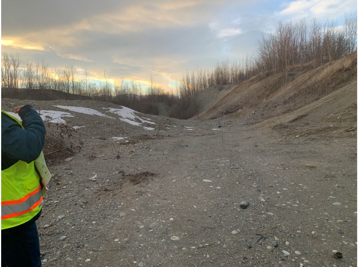
Looking south within the extraction area at the berms along the west and south sides
