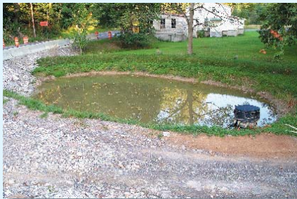
Small, temporary sediment traps intercept and detain construction site runoff so soil particles can settle out. Note how the outlet riser for this trap has been wrapped with filter fabric to increase detention time and trap suspended sediment. Designing traps and basins with long flow paths between the inlet and outlet also helps to increase sediment removal efficiency by extending the detention time. Where space restrictions prevent long basin designs, barriers placed in the basin can lengthen detention times by creating a serpentine flow path between the inlet and outlet.
