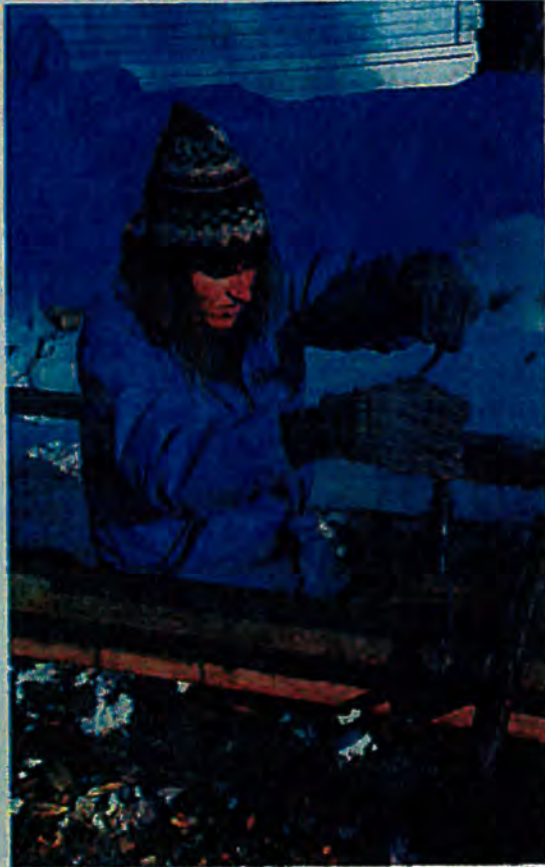
Above: Pam Robinson carefully sets up the guide to flatten one side of a 20-foot log being readied for a cabin. (Ron Dalby) Below left: By March, the cabin the Robinsons were building was almost ready for a roof. (Ron Dalby) Below right: In the kitchen of her Dalteli Lake home, Pam Robinson sets out jars of home-canned moose meat to cool. (Roger Robinson)
