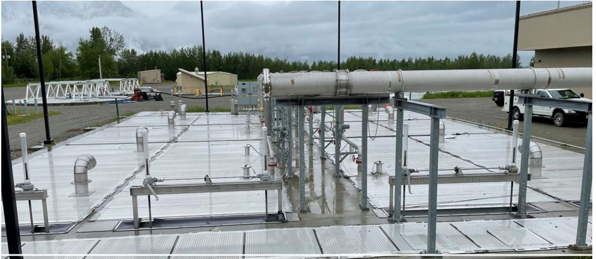
MBBR- Moving Bed Biological Reactor (2018)
