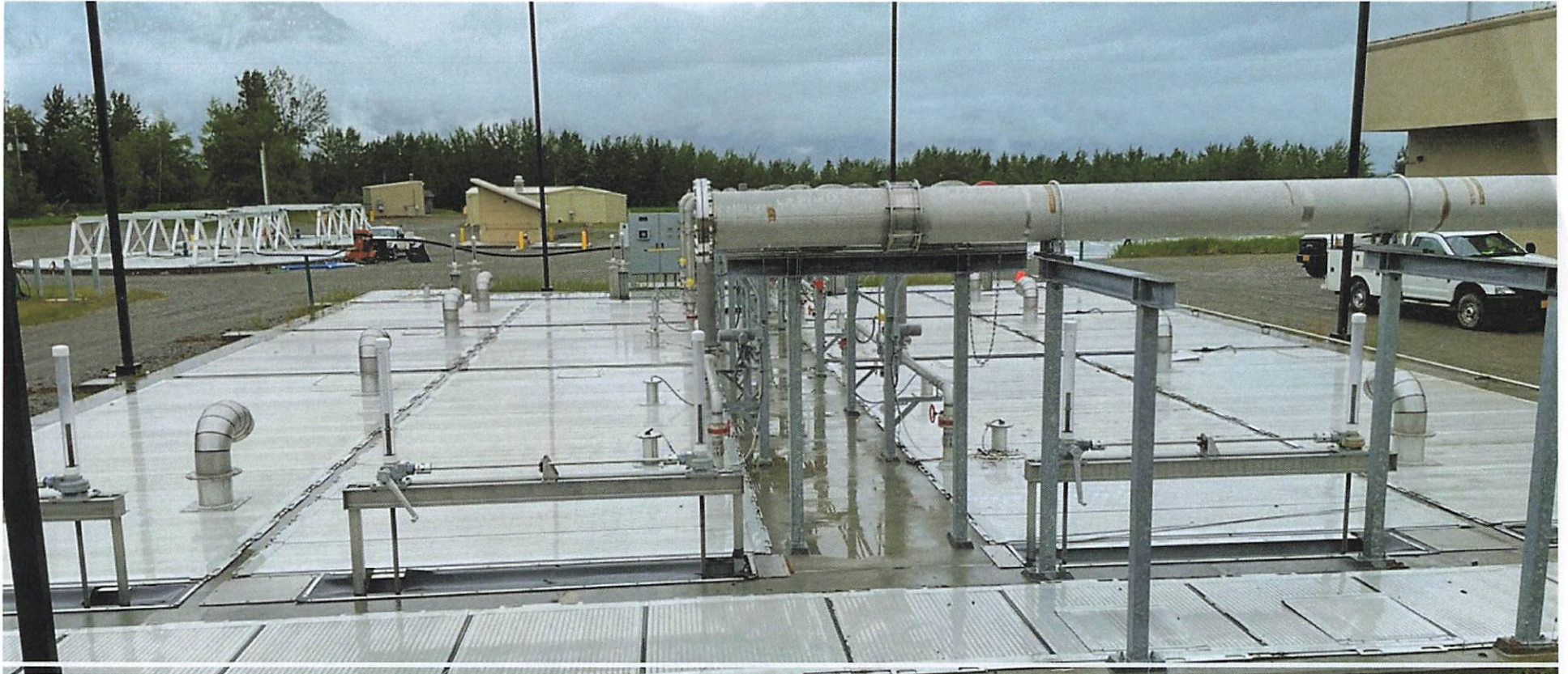
MBBR- Moving Bed Biological Reactor (2018)
